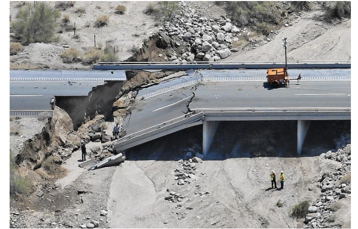
I-10 Washout in California, 2015
